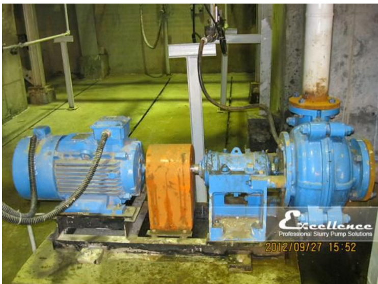
EHR-3C Copper-molybdenum Plant In Mid-East
