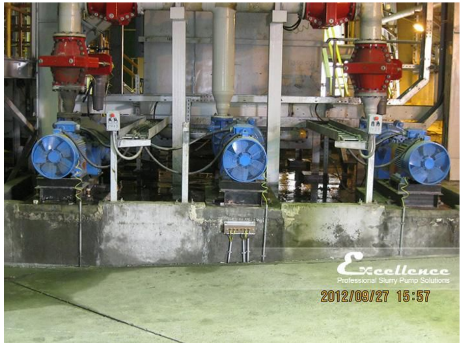
EHR-3C Copper-molybdenum Plant In Mid-East
