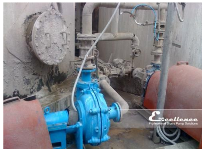
50EZ-A50 in Mid-East Sodium Silicate Plant
